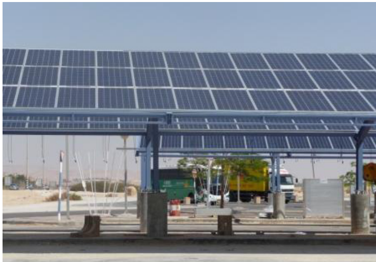
50 KWP installation at the Yotvata Parking Lot
