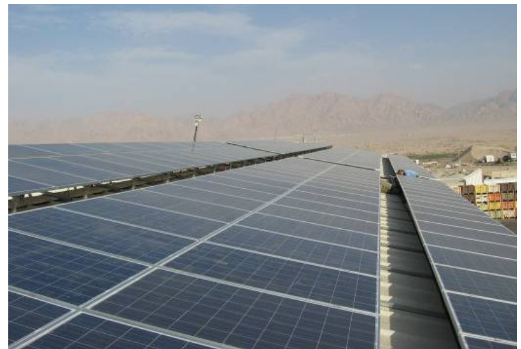
50 KWP installation at the Eilat industrial area
